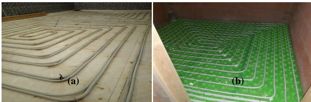
Figure 9. Description of existing central floor heating for the bathroom (Authors, 2023) (a): Medium performance heating; (b): High performance heating
