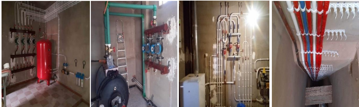
Figure 8. Illustration of materials and accessories for central heating of a residential building located in the city of Bechar (Authors, 2023)
