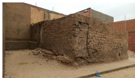
Housing in precarious initial state source :Authors 2021
